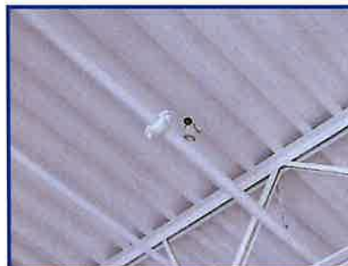
Typical Sprinkler Head
