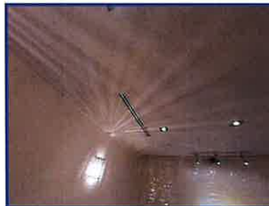
Pot Lights and Mounted Light Fixtures
