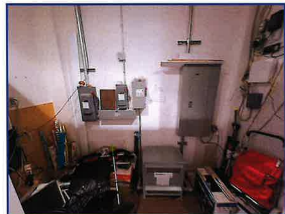
Mechanical Closet 200 Amp 600 Volt Electrical Service & 30 KVA Transformer
