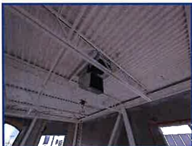
Roof-Top Hvac Unit
